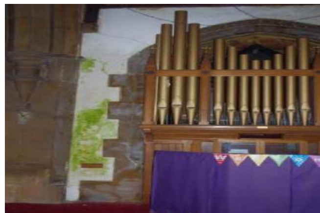
Green Mould on damp wall by Pipe Organ
